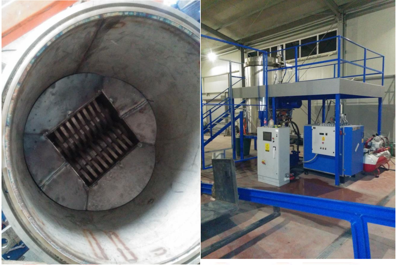
Picture.2 and 3. ARI-1100 system installed to Timisoara Medical waste sterilization plant
