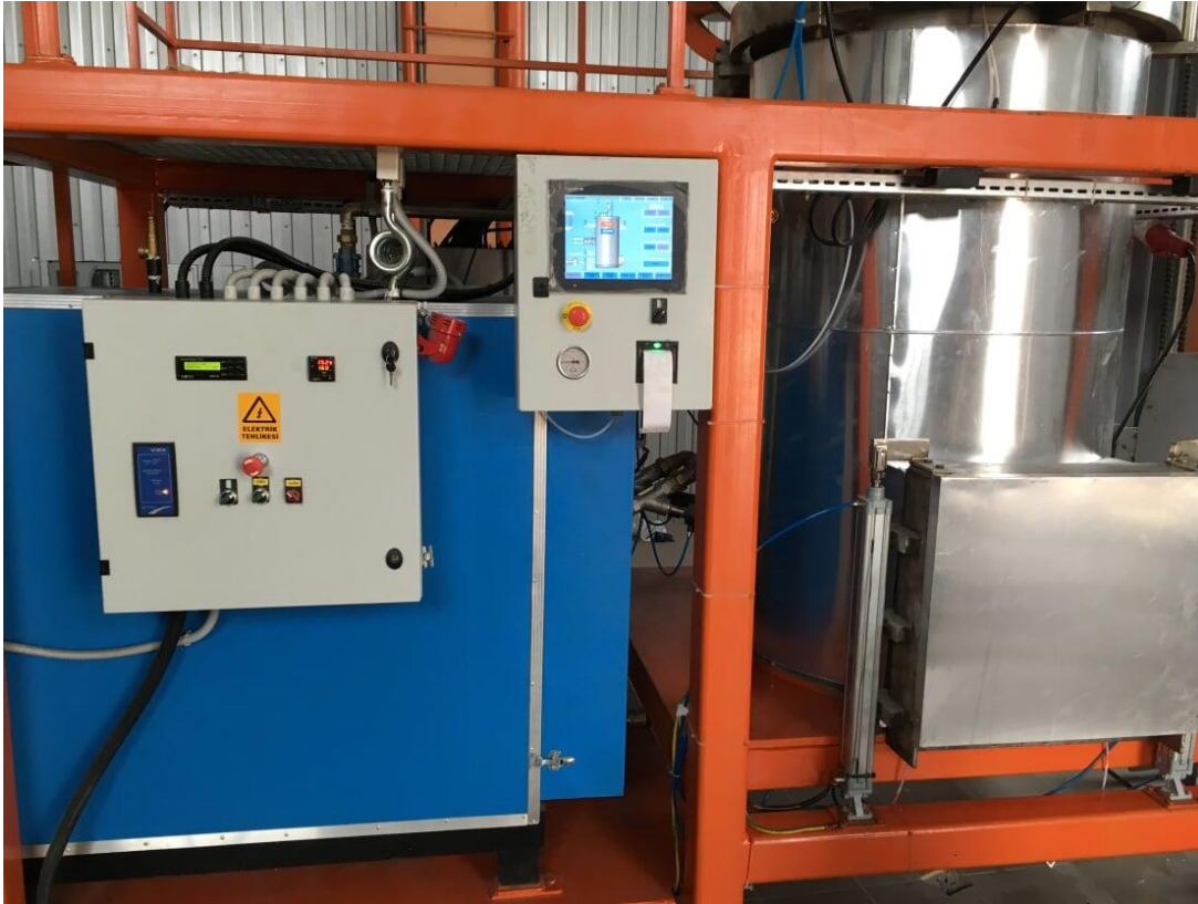
Picture.3. ARI-550 Installed in Chisinau
